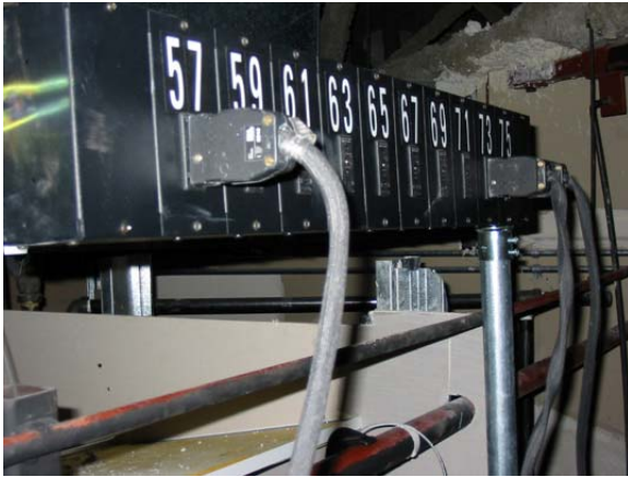
Power strip on batten
