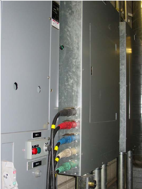
Correct power boxes
