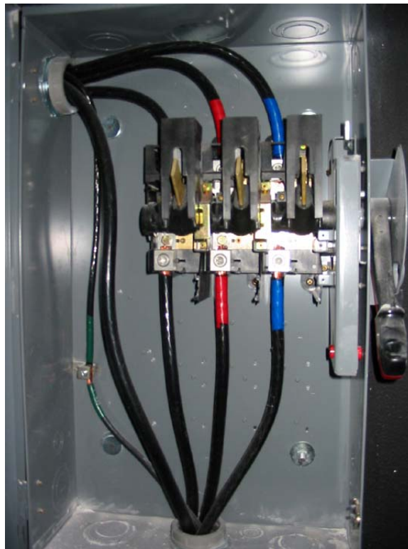
Box without cam locks (notice only 4 main wires)
