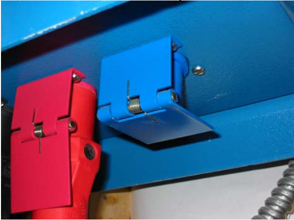
Bottom of box (cables will not be there)
